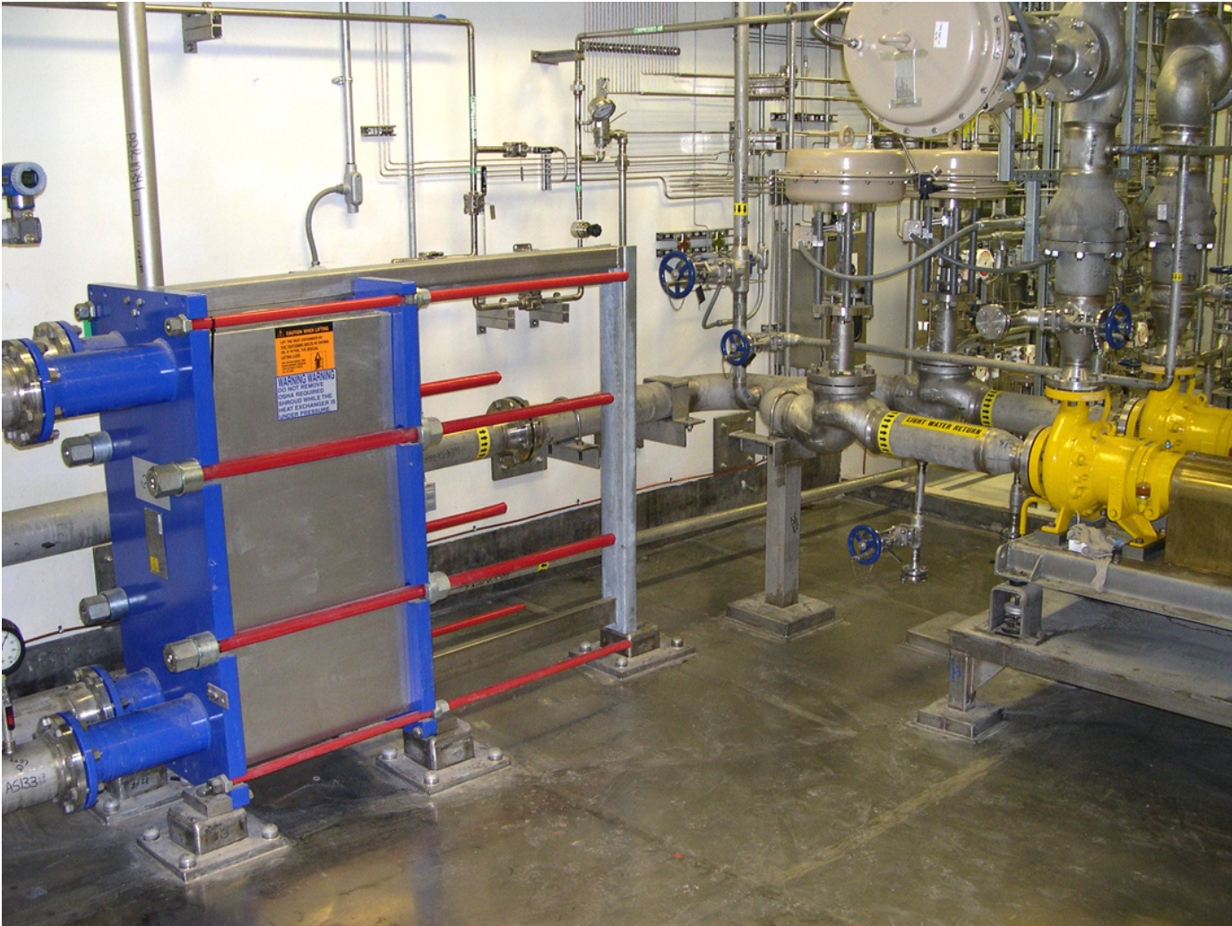
Plate type Heat Exchanger
